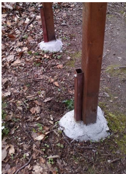
Fig. 3: Inappropriate anchoring of the wooden posts of the information board, structural protection is not ensured (Kotásková)
